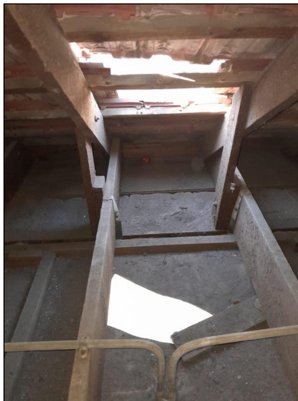
Figure 4. Roof and ceiling damage in Simon's Town
