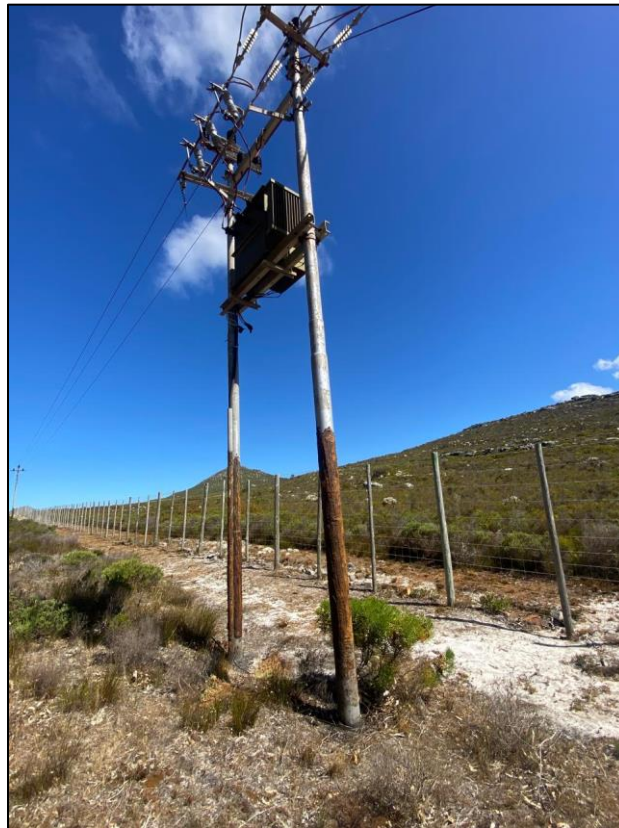
Figure 8. Greased electrical H Poles on Plateau Road
